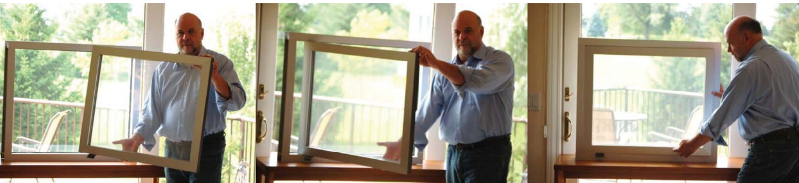
Figure 3. Single Low-E insert retrofit installation of the Low-E polymer film in front of the actual window.
